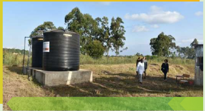
Rainwater harvesting system funded by NUFFIC
